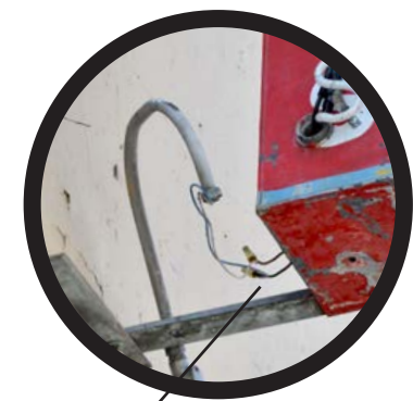
The exposed wiring outside of this sign cabinet is unsafe and non-compliant.
