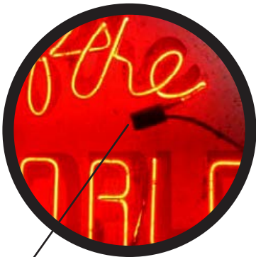
Rubber boots and wiring should never be outside of the metal cabinet as a repair shortcut on a vintage sign.
