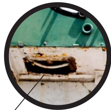
Exposed wire is unsafe. Unsealed access panel invites pigeons to nest. Bird guano will accelerate rust damage in the metal cabinet.
