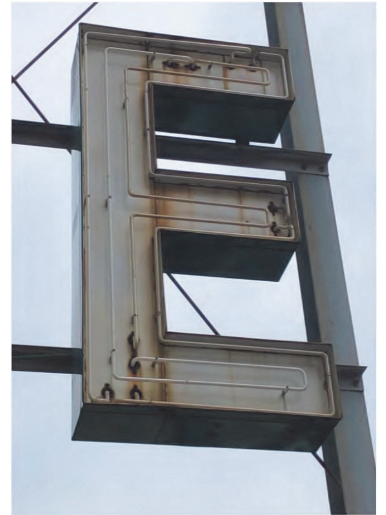
EXPOSED FOUR TUBE WHITE NEON MOUNTED TO INSET FACE, RUST AREAS TO BE CLEANED WITH STEEL WOOL.
