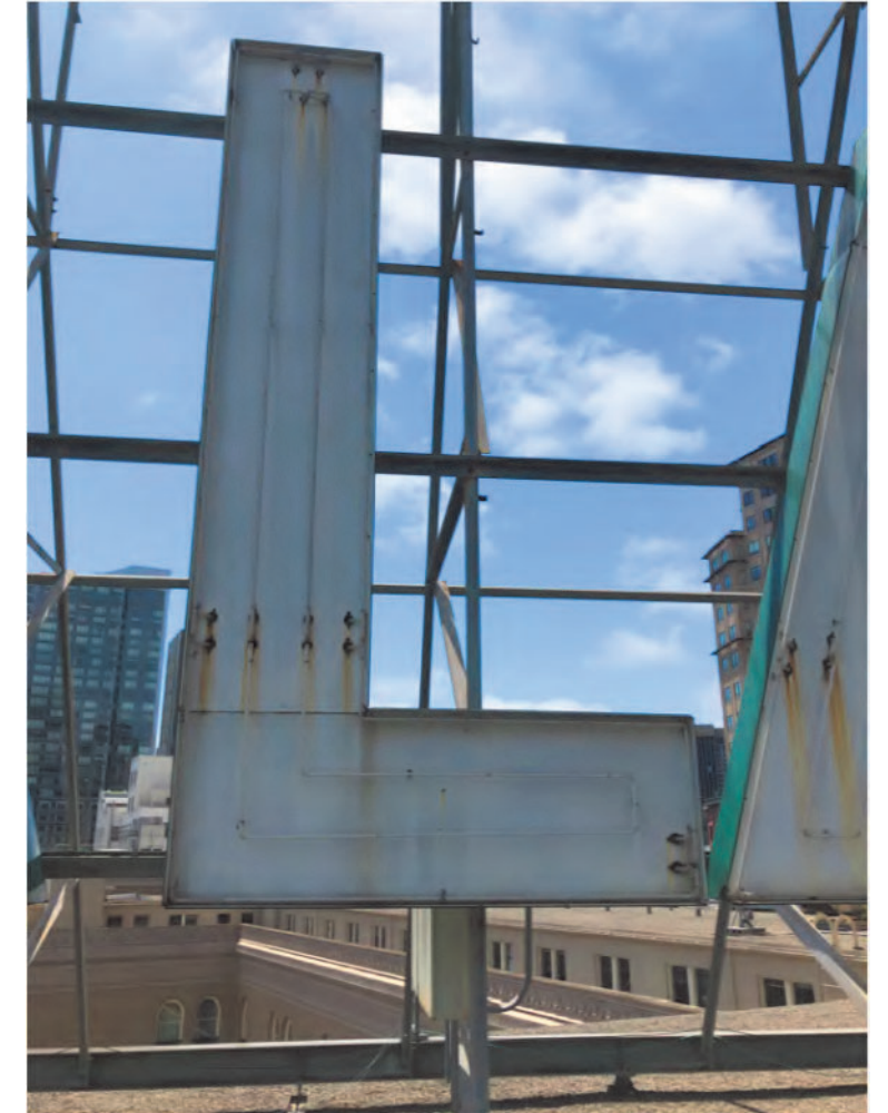
EXPOSED FOUR TUBE WHITE NEON MOUNTED TO INSET FACE, RUST AREAS TO BE CLEANED WITH STEEL WOOL.
